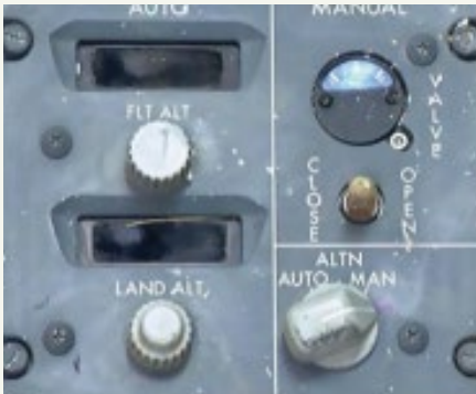
The pressurisation panel. The pressurisation mode selector can be seen at bottom right
