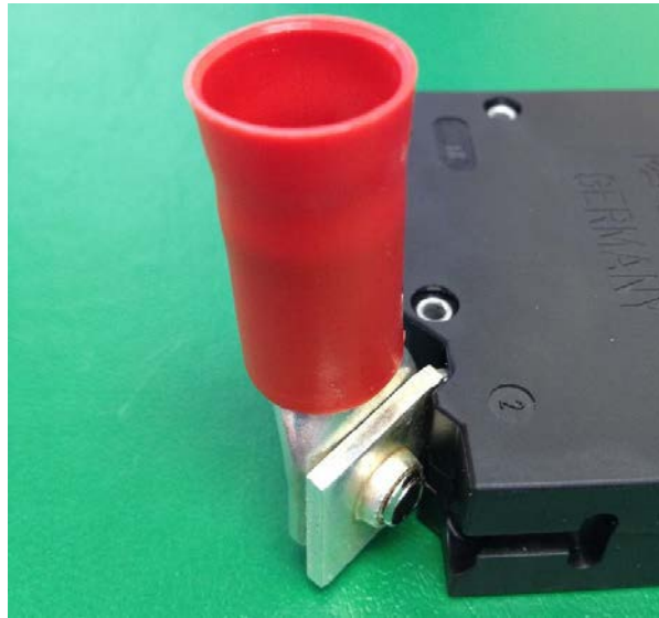
Figure 6 - Improperly crimped CB fitted to emergency medical equipment
