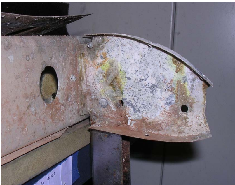
Figure 3. Missing rivets and rib corrosion.
