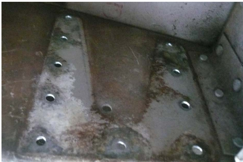
Figure 5. Corroded wing structure under the flap hanger bracket.
