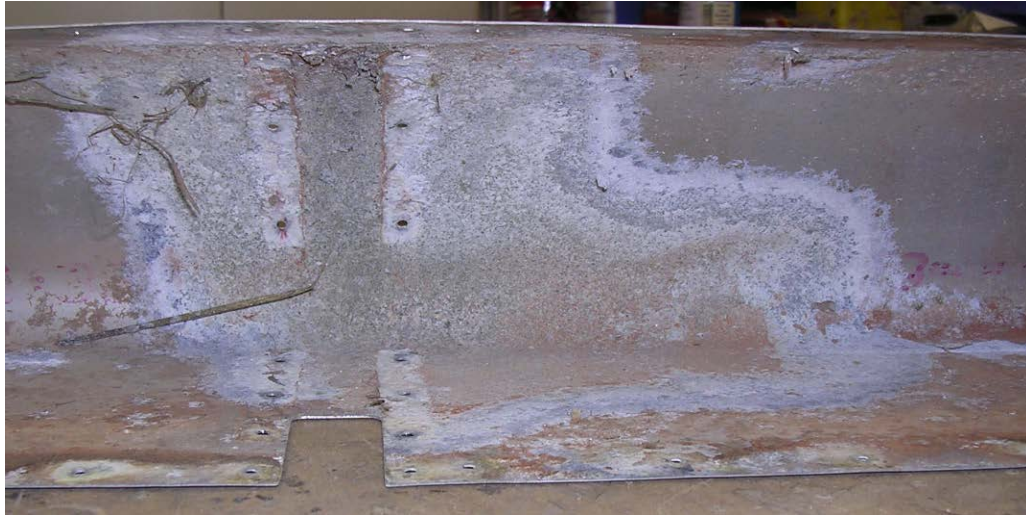
Figure 2. Removed flap skin showing extensive flap nose skin corrosion.
