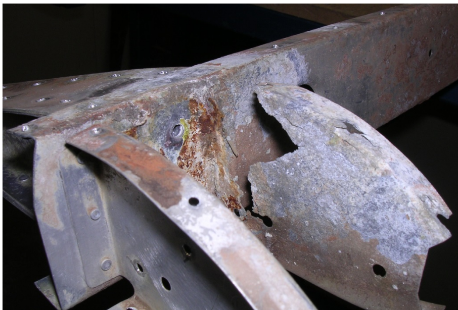
Figure 1. Typical flap nose rib and spar corrosion The steel hinge arm has been removed.
