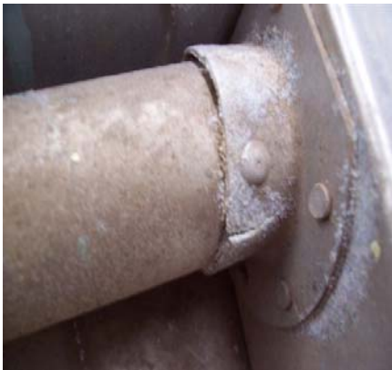
Corrosion in a elevator torque tube adapter on a CESSNA 172N
