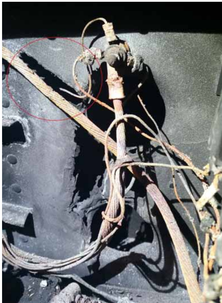
Figure 2 – Arc / fire damage to aircraft structure
