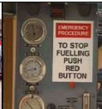
Refuelling vehicle emergency stop button
