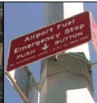
Refuelling hydrant emergency stop button
